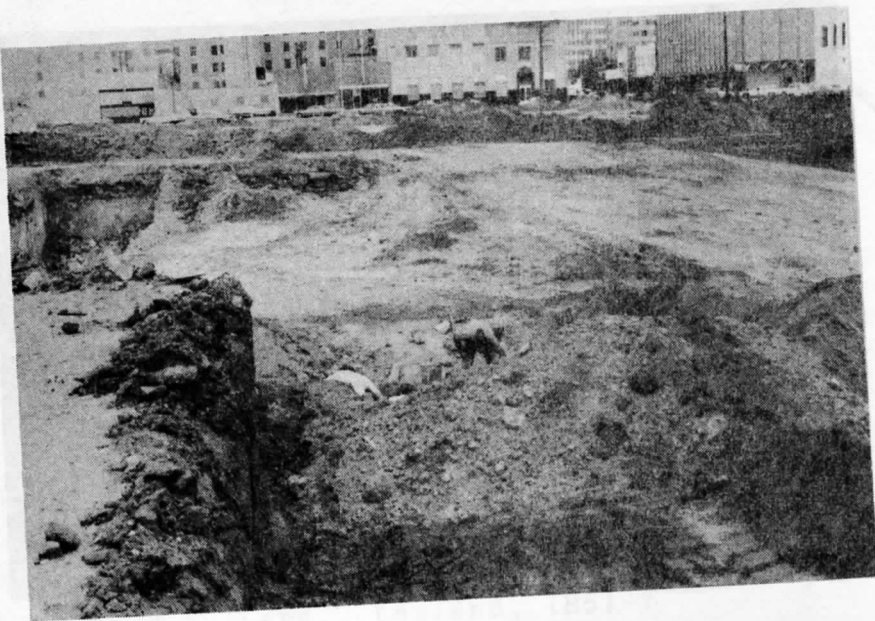
THE AREA OF THE FEDERAL BUILDING BASEMENT EXCAVATION AND WELL SITE VIEWED TO THE WEST.
